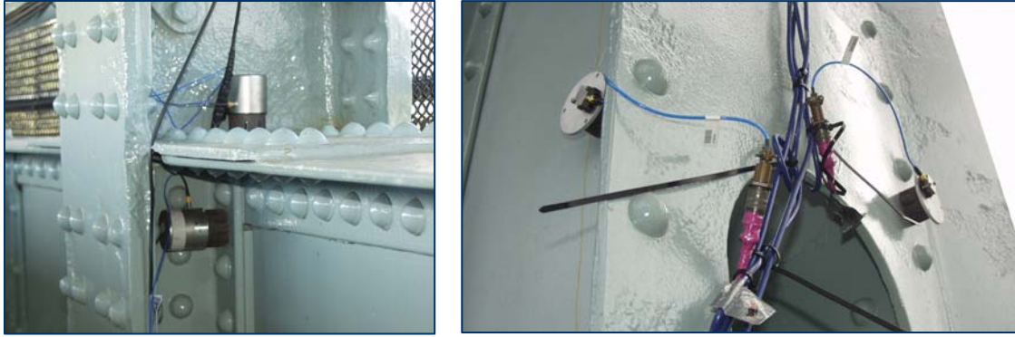
Figure 5-11 Vertical and transverse on the lower deck level of the arch span (left); Transverse and longitudinal sensors on the tower (Rigth)
